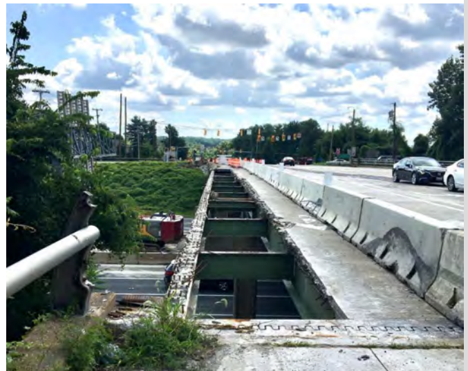
Crews are making progress on the demolition of the Georgetown Pike Bridge, as pictured above.
