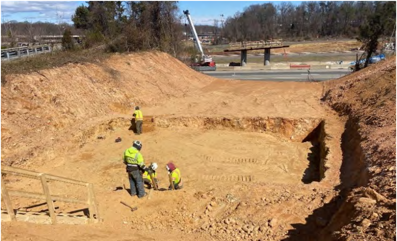
Workers prepare the site for pile driving at the southern landing of a new bridge over Dulles Toll Road. Starting in late March, a total of about 26 steel piles will be driven at this location, followed by a similar number of piles driven on the opposite side of the Dulles Toll Road, farther away from the Gates of McLean. The under-construction center pier of the new bridge is visible in the distance.
